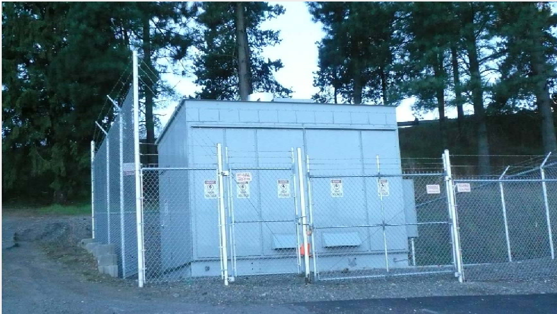
Prefabricated Traction Power Substation
